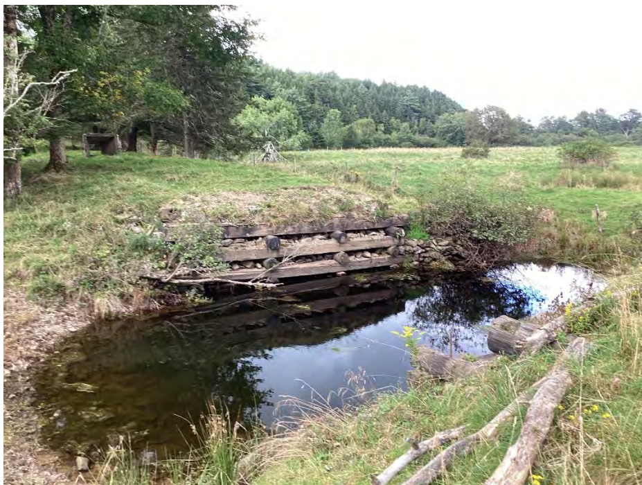
Image 8. Abandoned road infrastructure at Cross Roads, Stewiacke.
