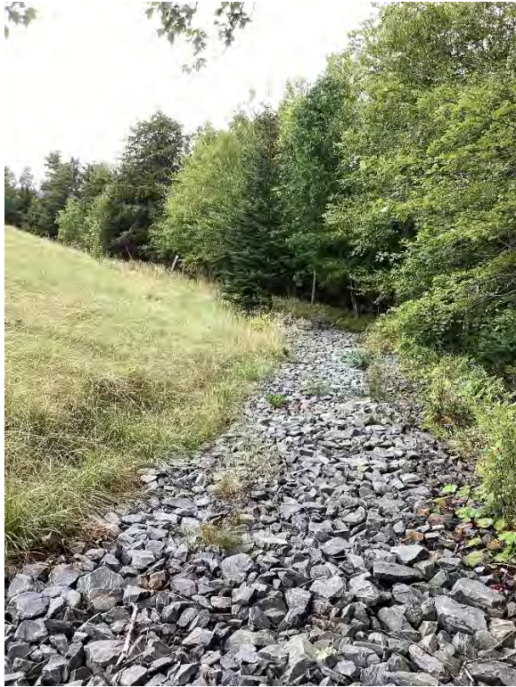
Image 9. Gravel berms for mitigation of off-site movement of landfill sediments.
